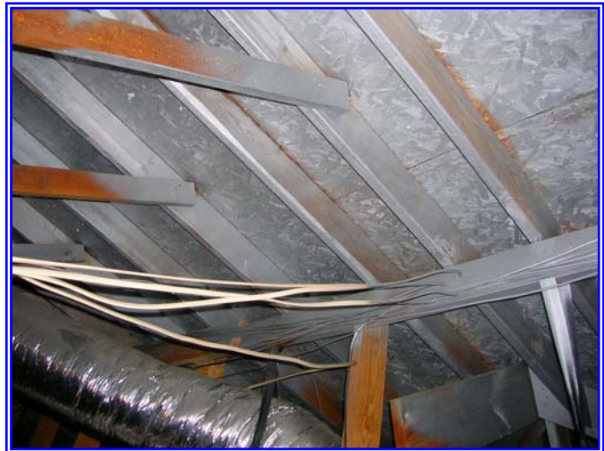
OSB ROOF DECKING WITH RADIANT BARRIER PAINT
