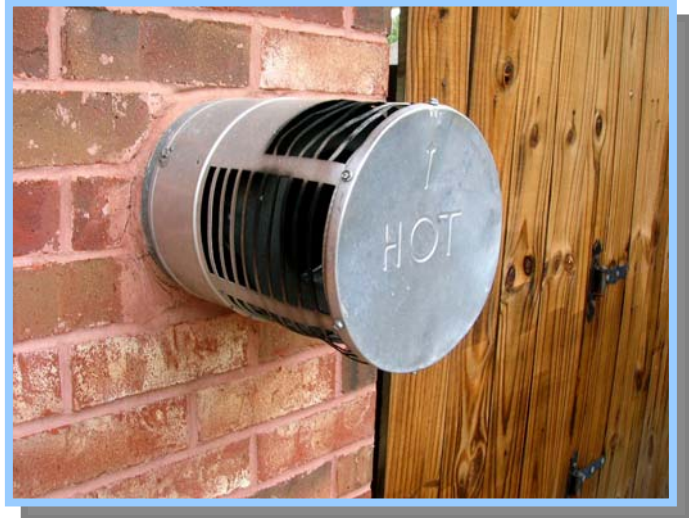
DO NOT COVER THE EXTERIOR VENT
