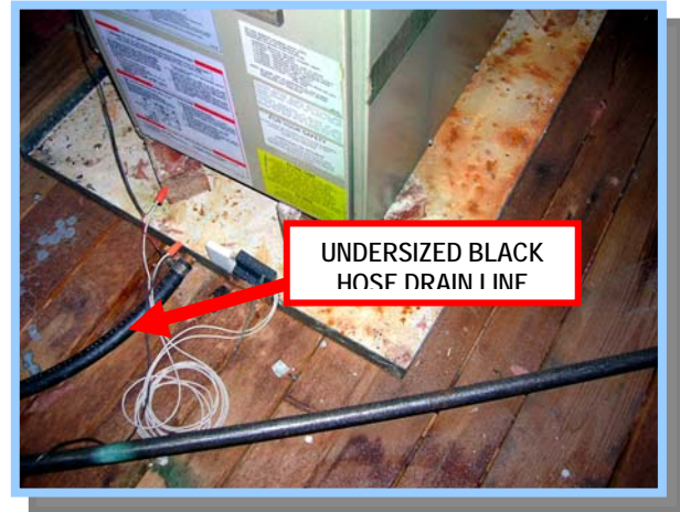
RUSTING DRAIN PAN UNDER 2 ND FLOOR UNIT
