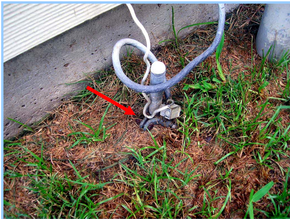
WRONG TYPE CLAMP AT EARTH GROUND ROD
