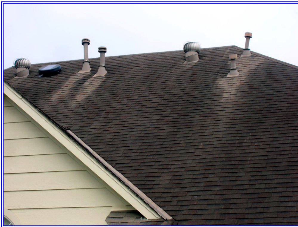
DARK STAINS ON THE AGING SHINGLES
