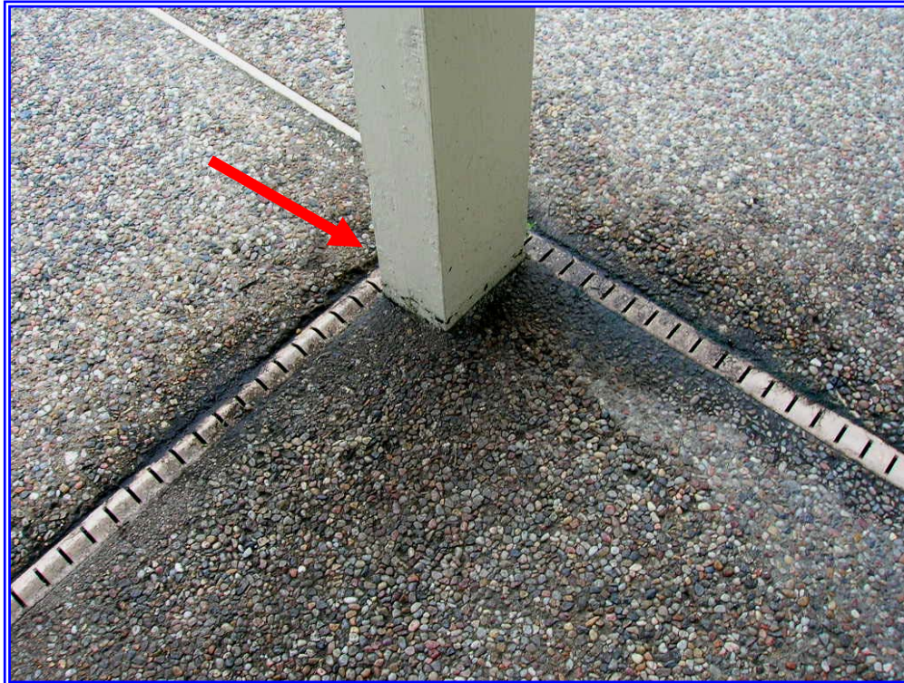
WOOD POST MAKING CONTACT WITH PATIO CONCRETE
