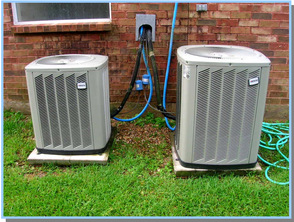
A/C CONDENSING UNITS
