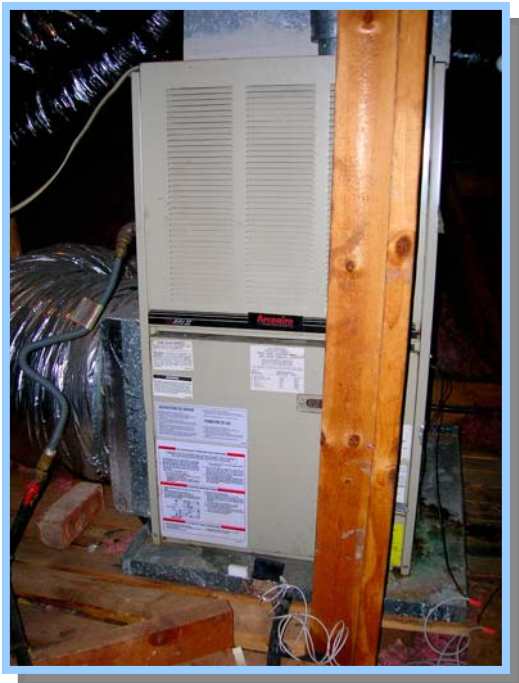
1 ST FLOOR GAS FURNACE
