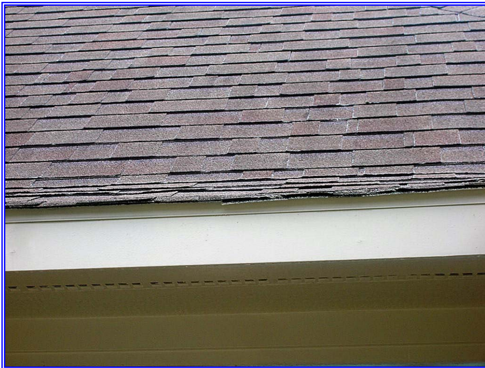
EXPOSED FIBERGLASS MATT AROUND THE EDGE OF THE SHINGLES
