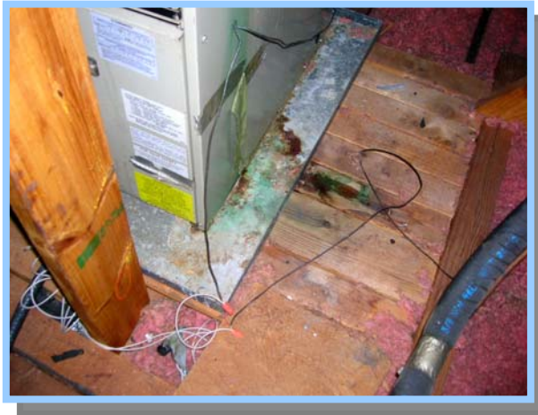
DIRTY DRAIN PAN UNDER 1 ST FLOOR UNIT
